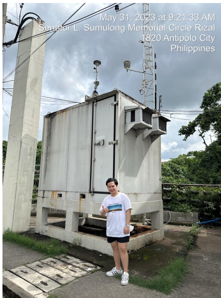
Figure 13: DENR Equipment inside the Container Van
